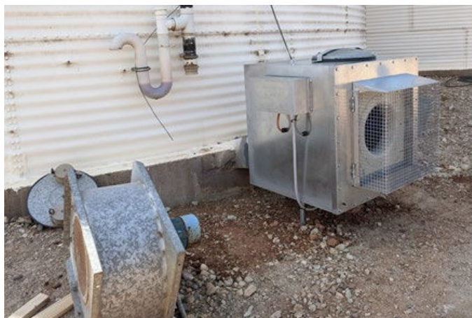
Figure 13. Original 3 kW fan (left) and new 5 kW fan (right)
