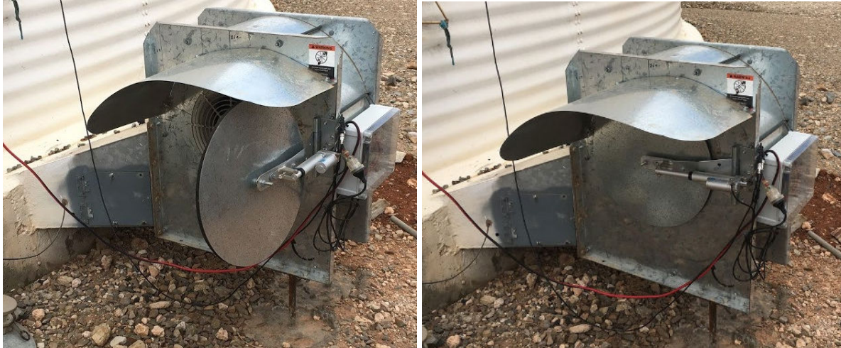
Figure 19. Electric actuated door to seal the fan inlet during periods of higher temperature. Door open (left) and door closed (right)
